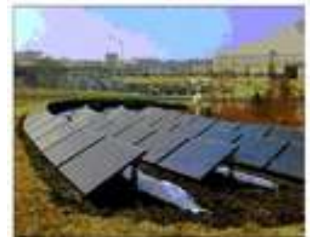
Pentagon's Ground Mounted 30 kW PV System Showing 4 Acres of PV Modules
