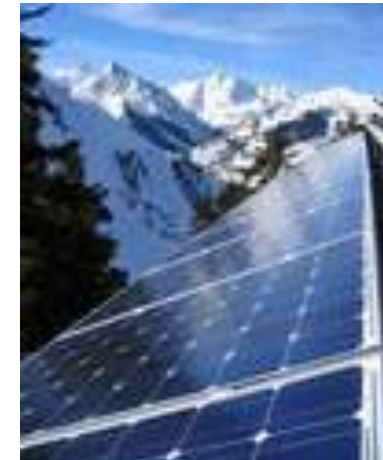
PV System at Aspen Mountain Ski Resort
